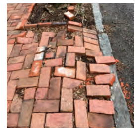
If your sidewalk poses a tripping hazard, let us help you fix it.
